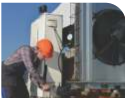
AIR CONDITIONING DESIGNING & CONTRACTING SERVICES
